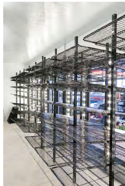
Standard Shelving Installed
